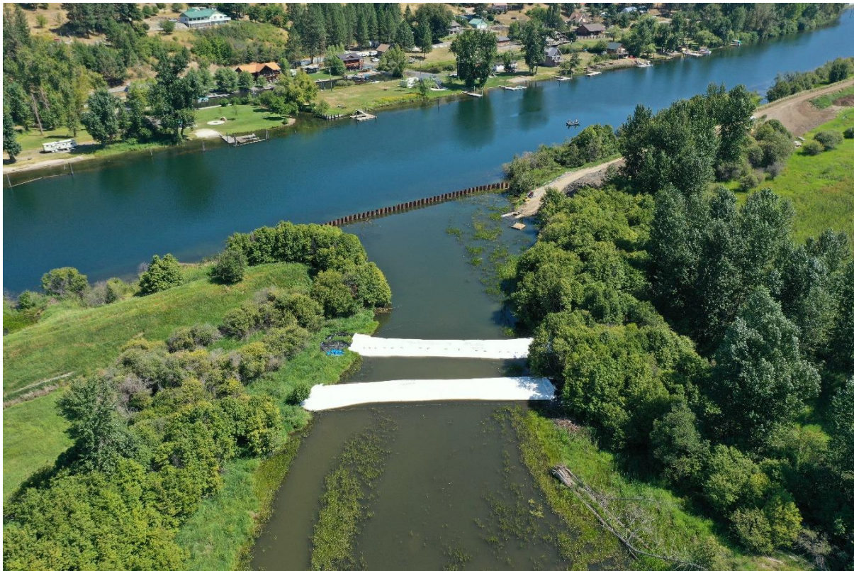
Sheet pile and inflatable coffer dam installation at the Hepton levee breach (July 2023).
